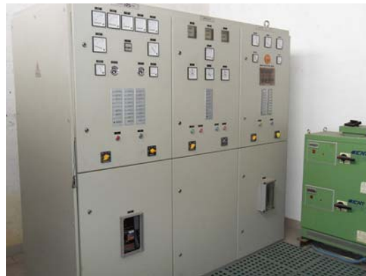
Electrical Switch Gear
